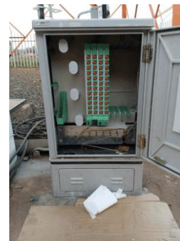
Outdoor ODF Installation
