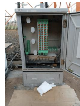
Outdoor ODF Installation
